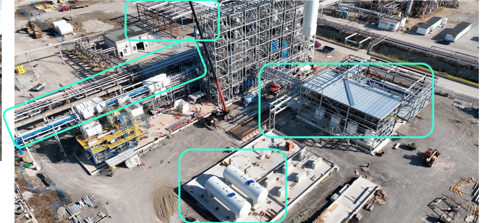
“After”: Clockwise from top we see the biomass building, HTC building and filter press, solvent tanks, piping modules
