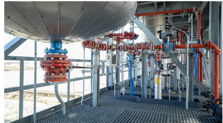
Key production module showing process equipment. The newly fabricated pipe rack modules are designed to interconnect the plant's key production modules
