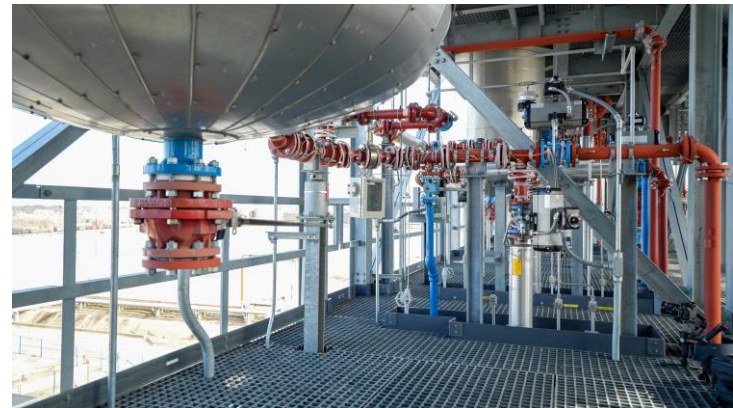
Key production module showing process equipment. The newly fabricated pipe rack modules are designed to interconnect the plant’s key production modules
