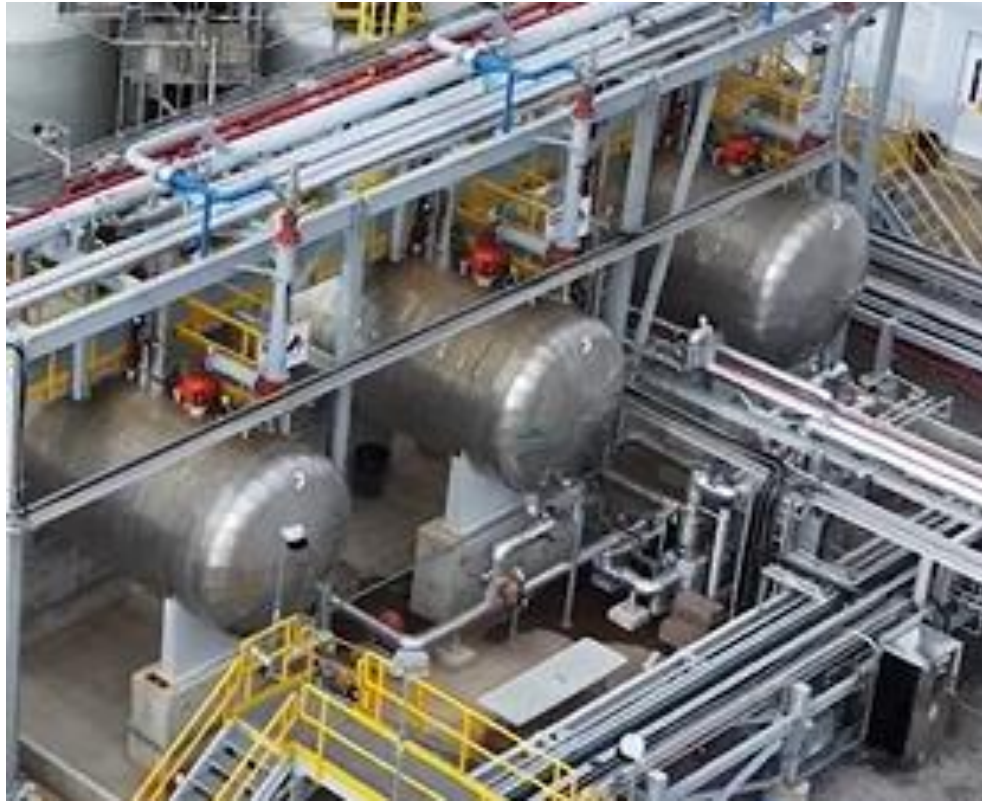
CMF storage tanks at Origin 1 in Sarnia, Ontario, Canada.
